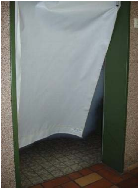
FIGURE 3: Influence on the characteristic of the fresh air flow into the fire compartment by a PathMaster ® with the curtain nearly covering the whole opening and forcing the fresh air flow to go in low.
